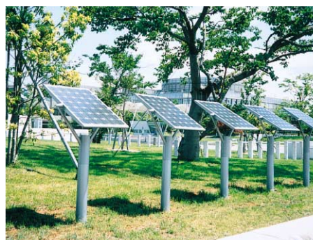
Kurobe Plants solar electricity generation system
