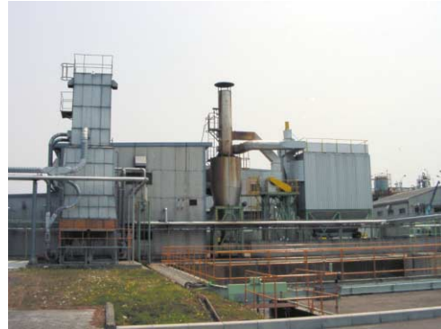
Tohoku Plant equipment used to capture the heat energy of burning wood scraps
