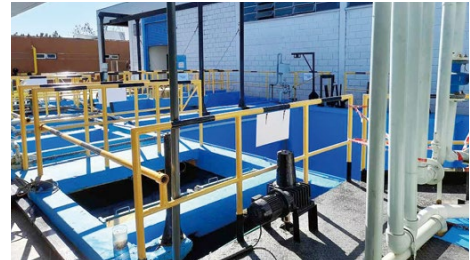
Wastewater diagnosis setup
